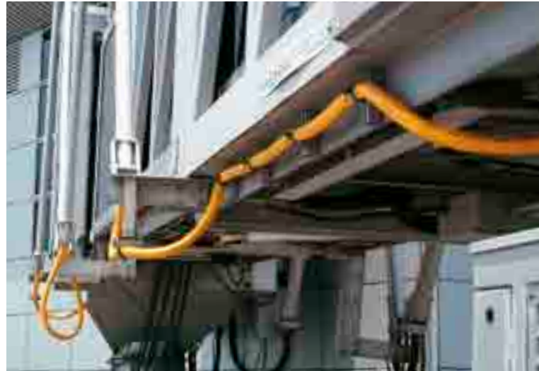
Kuala Lumpur International Airport, BETAjet® 400 FRNC-smartflex-V cable
